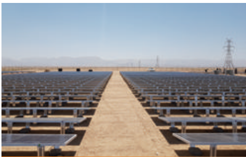
Project Size: 1.5MW Installation Site: Pakistan
