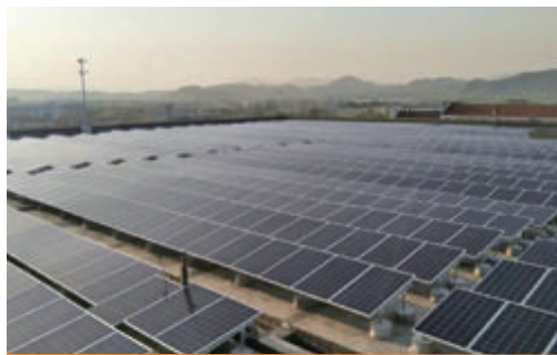
Project Size: 3MW Installation Site: China
