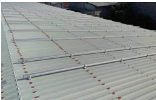
Project Size: 2MW Installation Site: Vietnam
