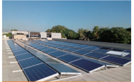
Project Size: 650KW Installation Site: UAE
