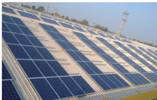
Project Size: 2.1MW Installation Site: India
