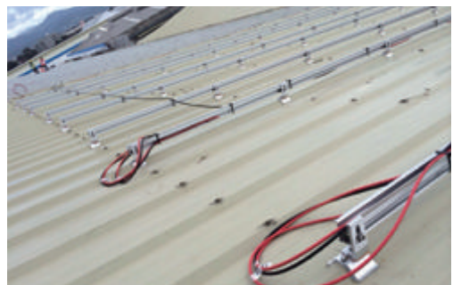
Project Size: 3.45MW Installation Site: Philippines
