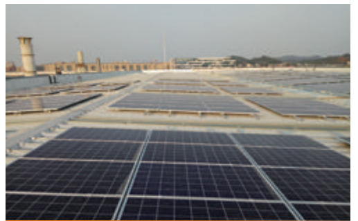
Project Size: 2.8MW Installation Site: China
